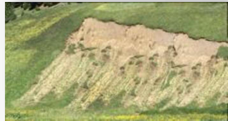
Figure 1: Significant disruption of slope surface stability
